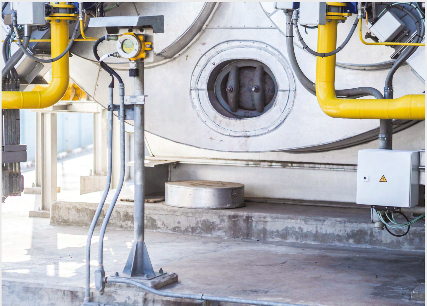
Fig. 1. Gas detector located outdoors in a hydrogen use area
